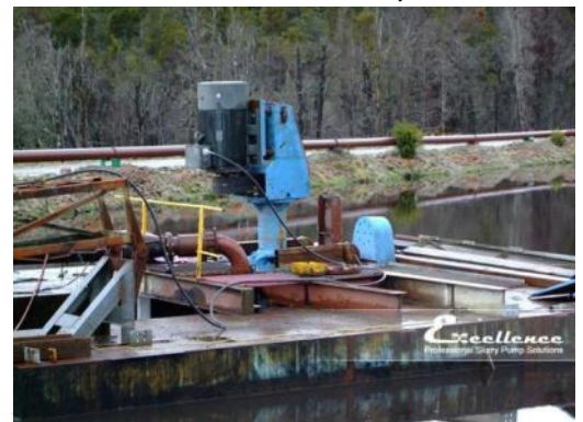
EVHM-6SV in Coal Washery in Australia
